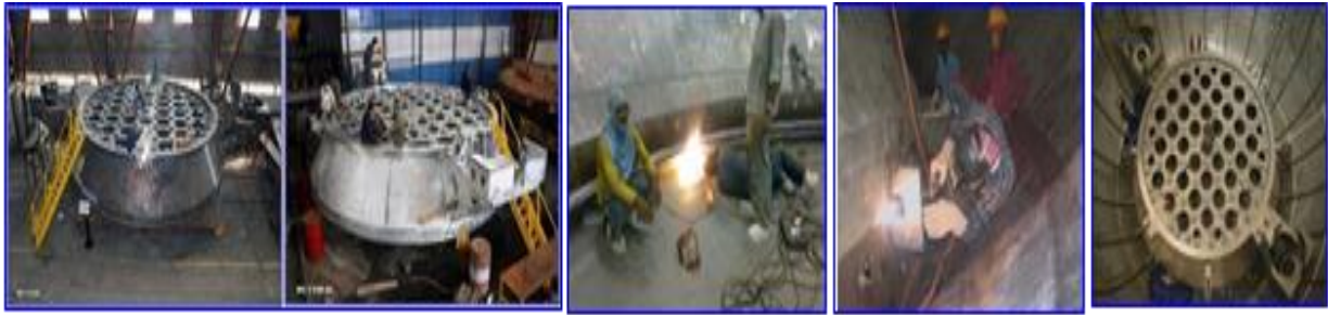
Figure-6: Welding and fabrication of Core Support Structure and integration with MV
